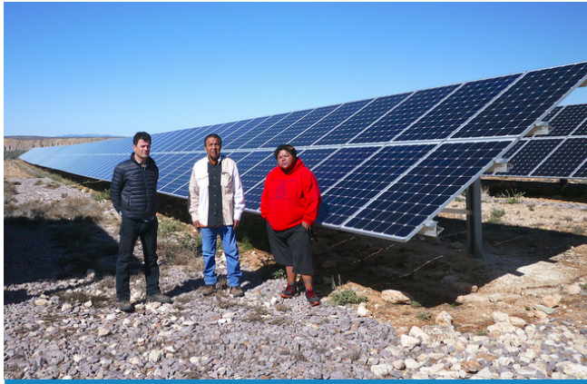
Regional Administrator Jared Blumenfeld, Tribal Council Member and Environmental Director Tommy Siyuja, Sr., and Augie Hanna visit a new solar array at the Havasupai Tribal School. This array will help save the Tribe money and energy, prevent frequent outages, and reduce greenhouse gas emissions. CREDIT: EPA
